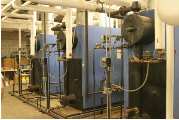
Boilers used for heating kitchen & new jail hot water year round
