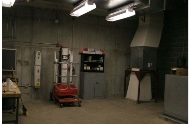
Location of new jail hot water solar storage tanks
