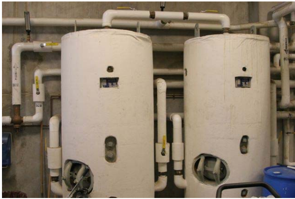
hot water tanks used for new jail hot water
