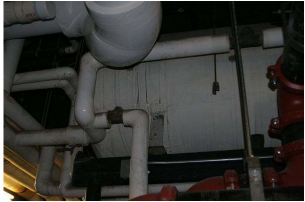
Boiler room 0016 hot water tank
