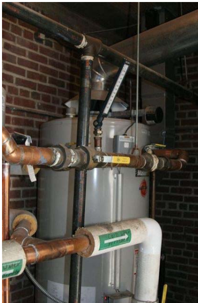
Boiler room 0016 hot water heaters
