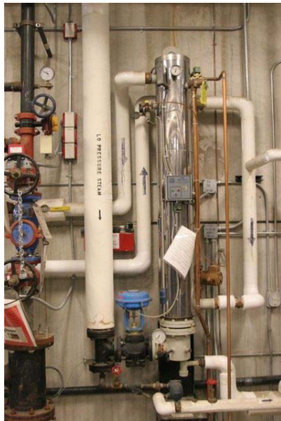
Heat exchanger used for new jail hot water
